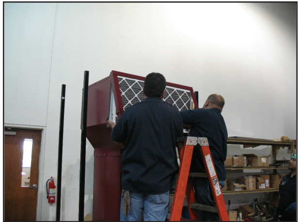
Install two odor ban carbon pleats in front of the exhaust panel filters.
